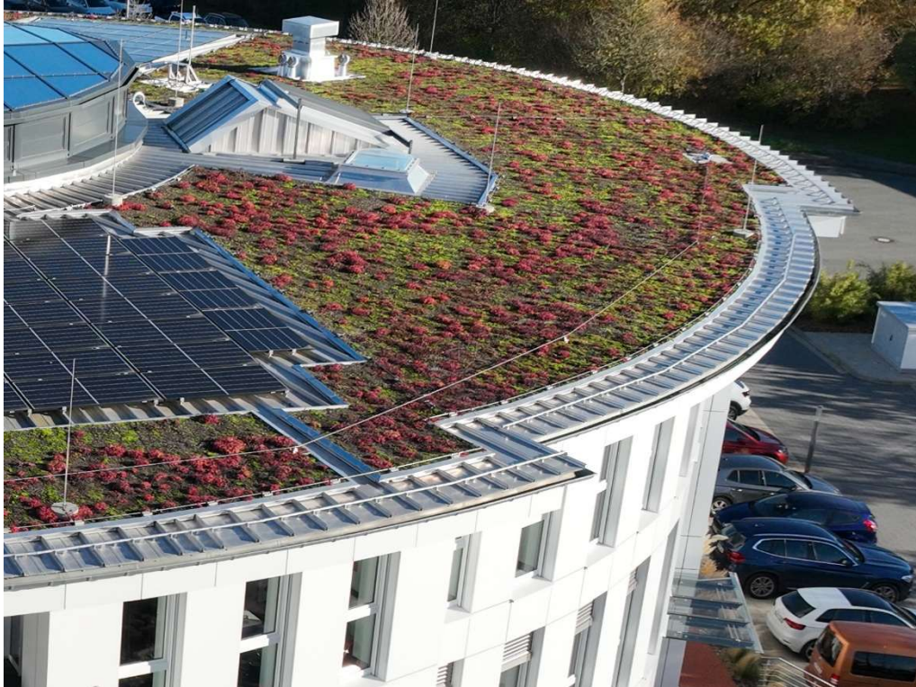
The green roof improves the microclimate, binds fine dust, and contributes to the natural temperature regulation of the building. Photo: Zambelli Holding GmbH.
